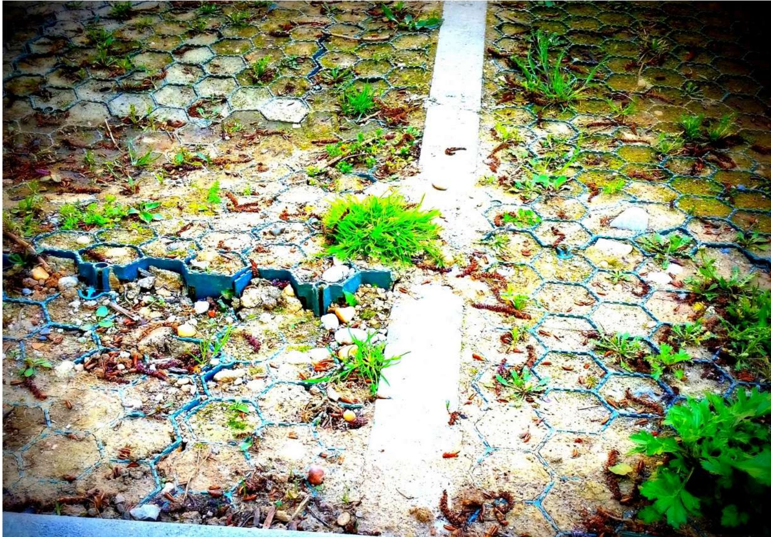
Parking perméable endommagé © Cherqui, 2015
