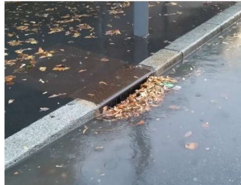
Blocked inlet © Cherqui, 2014
