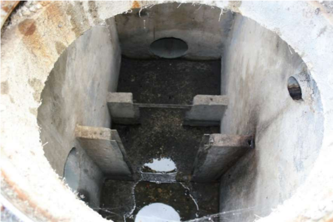
Inflow sabotaged (missing valve) © Bourgogne, 2010
